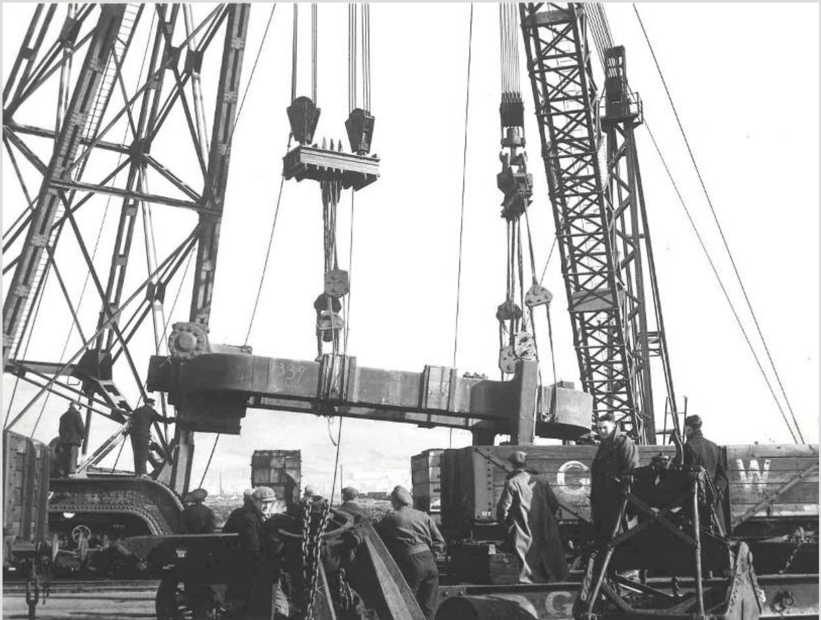
Piece of machinery weighing approx 120 tons
