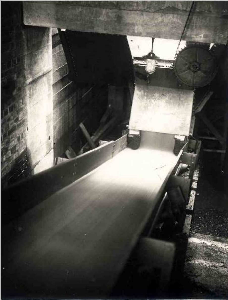
Conveyer used to take the coal from the hopper
